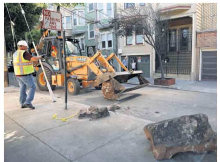
In this Monday, Sept. 30, 2019, photo, a San Francisco Public Works crew removes boulders from a sidewalk along a street in San Francisco, Monday, Sept. 30, 2019. In this Monday, Sept. 30, 2019, photo, a San Francisco Public Works crew removes boulders from a sidewalk along a street in San Francisco, Monday, Sept. 30, 2019.
